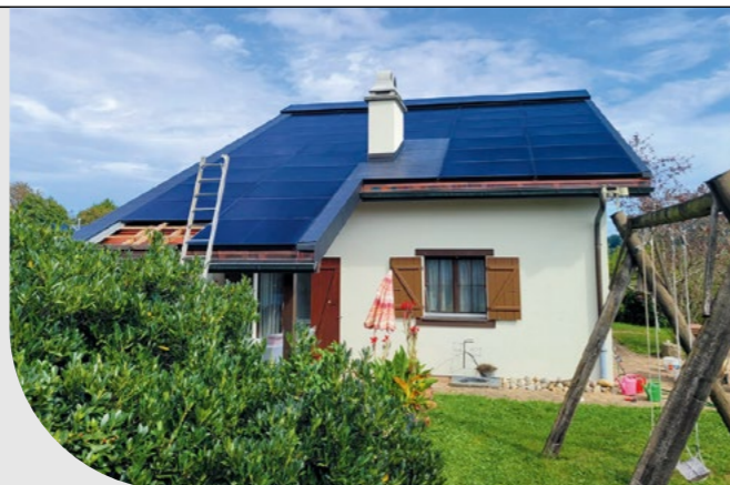
Installation Michel Plomb, Develier
