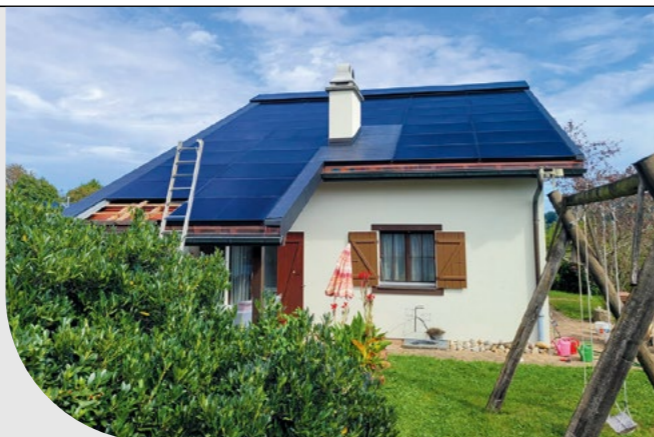
Installation Michel Plomb, Develier
