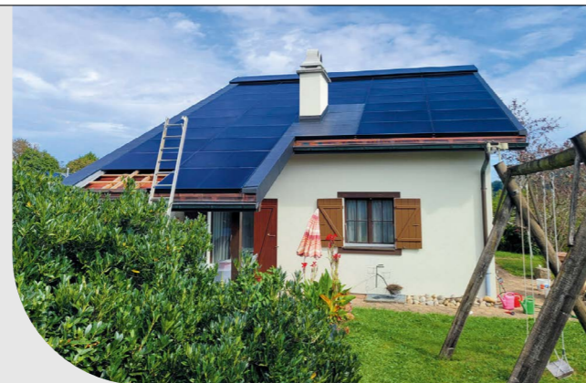
Installation Michel Plomb, Develier
