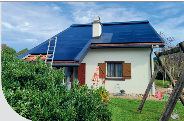
Installation Michel Plomb, Develier
