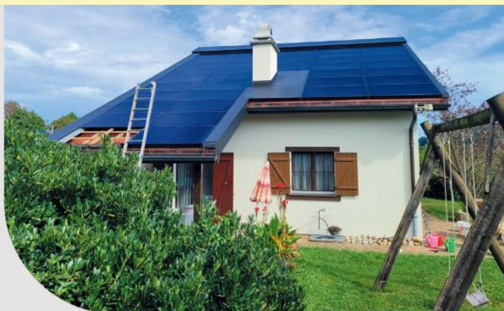
Installation Michel Plomb, Develier
